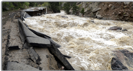
Above: Destroyed road in Boulder, CO - courtesy Daily Camera
