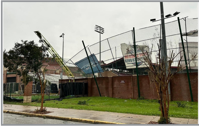
Damage to Dick Howser Stadium at FSU (source: @Greg Tish )
