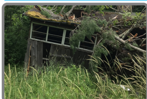
Damage from a tornado in New Hampshire in June. Credit: NWS GYX
