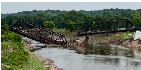
Floodwaters on the Big Sioux River collapsed a railroad bridge in mid June. (Credit: M. Widhalm)
