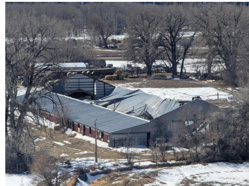
Collapsed barn roof near Columbus, Montana.
