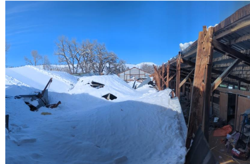
Snow load, locked in place by a low of -27^{\circ}\text{F} ( -33^{\circ}\text{C} ), led to this barn roof collapse on February 18.
